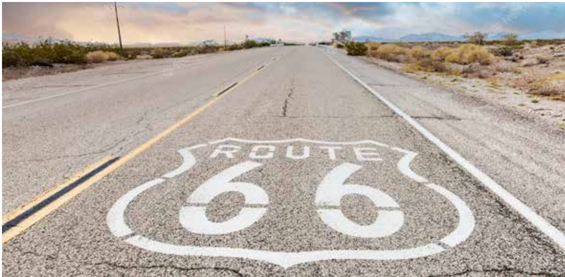
Fig 3: Shoving on turning point
