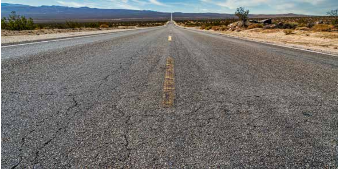
Fig 2: Alligator cracks in Flexible Pavement
